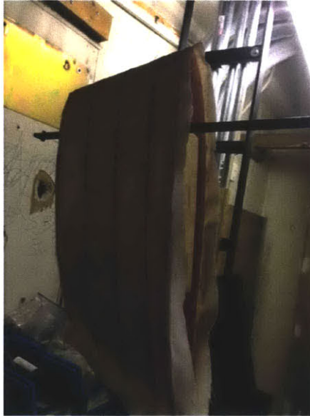
Figure 13: One of the forward struts hanging up to dry after its epoxy coat
