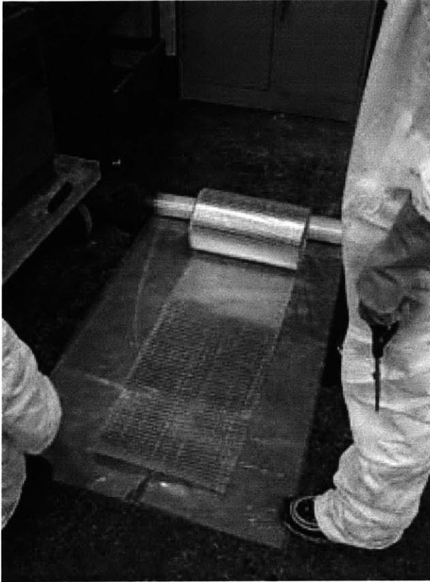
Figure 4.1 Tyfo® SEH-51A uncured fabric ready to be trimmed to size for installation
