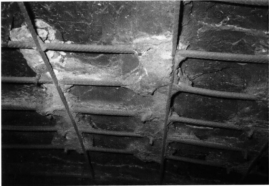
Figure 1: Thermal spalling effects on The Chunnel tunnel after the Nov. 1996 fire. (photo courtesy of The i-Center for Infrastructure Science and Technology, MIT)
