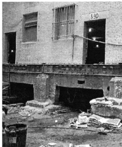
Figure 10 – Example of exposed footings from L.A. City Hall, CA.
