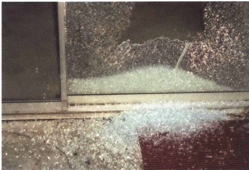
Figure 8 - Broken Fully Tempered Glass
