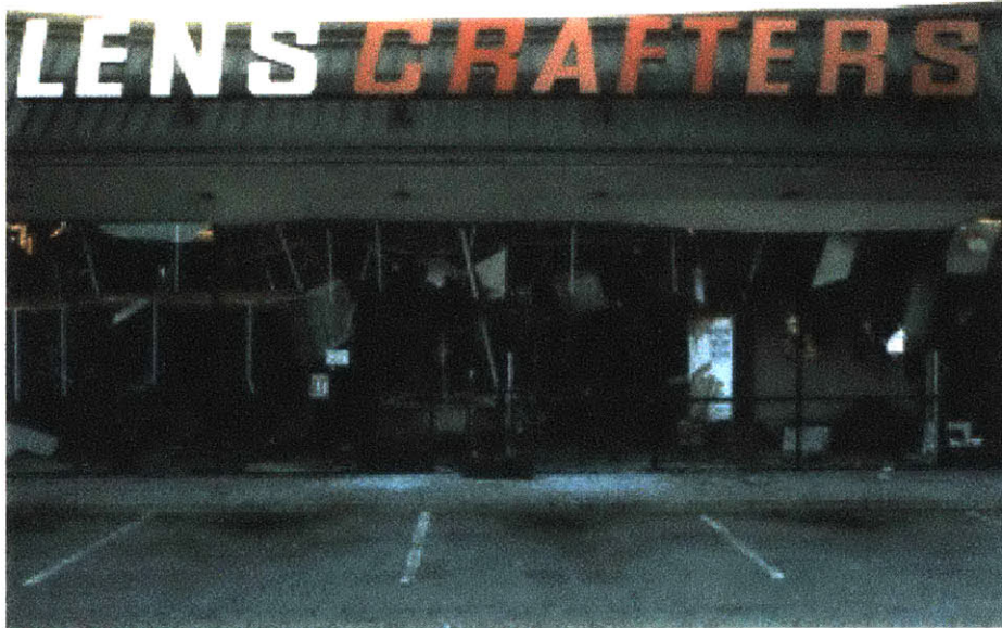
Figure 1 - Glass Storefront Damage following Loma Prieta Earthquake (Solutia, Inc., 2001)
