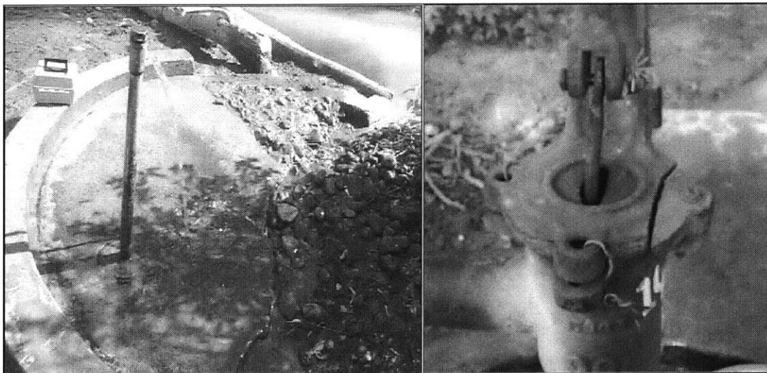
Figure 3-1. A Broken Platform and A Broken Handpump
