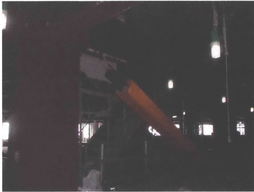
Figure 3-1: A hysteretic damper installed in a 44-story building.
