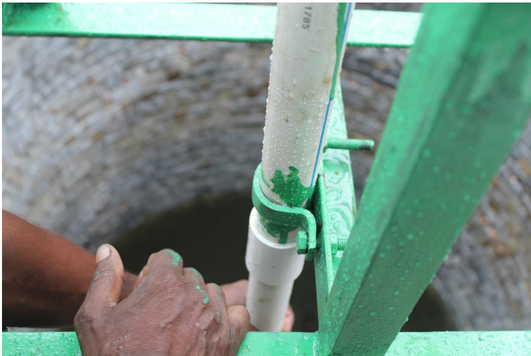
Figure 4.34. Connecting and gluing the long pipe to the piece of pipe supported by a clamp to the main structure.
