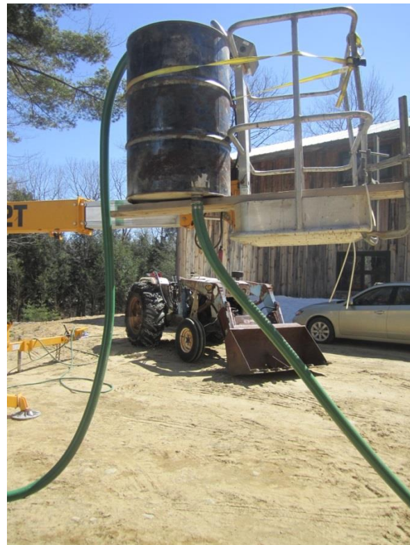
Figure 2.5. A makeshift funnel was created by strapping an oil drum to the back of the bucket lift.
