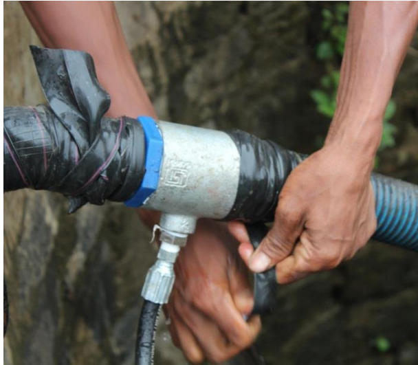
Figure 2.15. Wrapping rubber from used bicycle tires around the pipe fittings to eliminate leakage.
