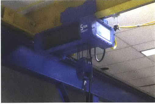
(a) Indoor Crane
