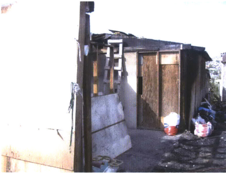
Figure 3.31 Remnants of burnt house
