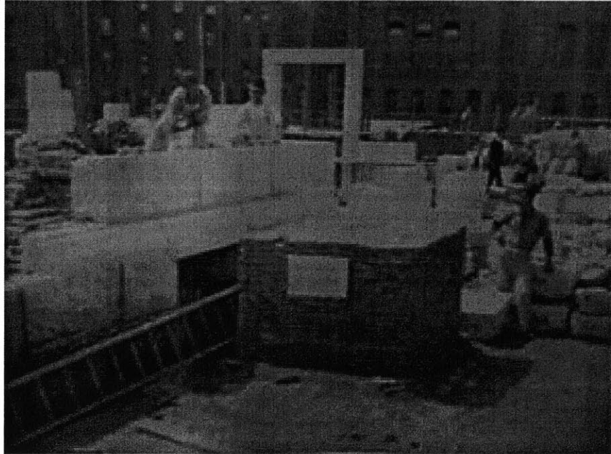
Figure 3.3 Tile arches loaded, April 20, 1889 (No. 60, Archives of the Trustees of the BPL)
