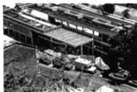
La Franja, San Agustín del Sur, Caracas, 1990. Built Part of the Project by the Author
