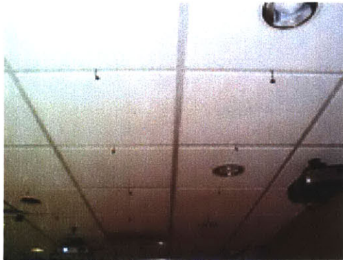
2.1.b – Array of microphones in the ceiling of the Intelligent Room
