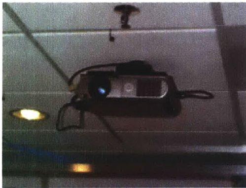
2.1.d – Projector mounted to the ceiling, which projects a display onto the opposing wall.
