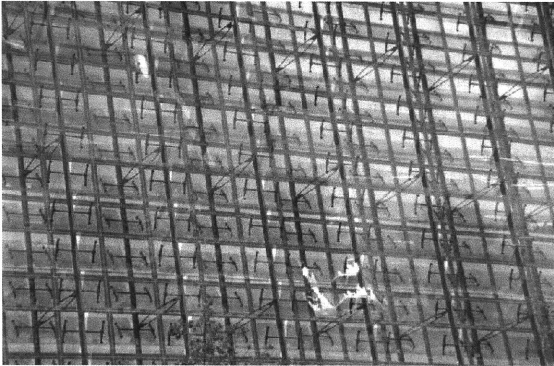
Figure 5 Operable exterior glass plates of double-skin facade for a bank in Munich
