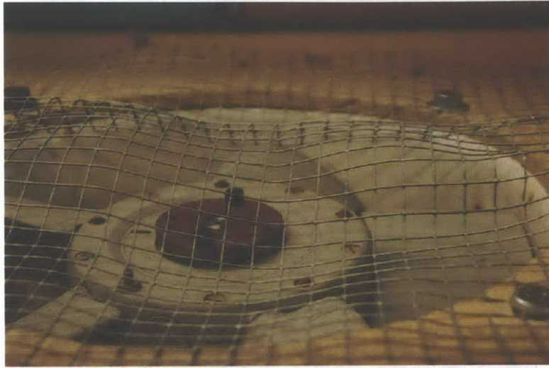
Fig. 5-2: A top view of the intake ventilation fan with no imbalance.
