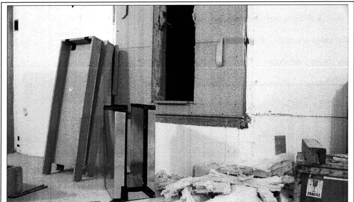
Figure 3.3 – Test section (seen from the source room) during installation of the U-shaped duct.
