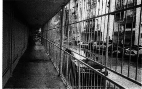
Fig 3.18. Fenced-in corridor accessing beauty salon from public parking; note residential building and parking on the other side of the fence.
