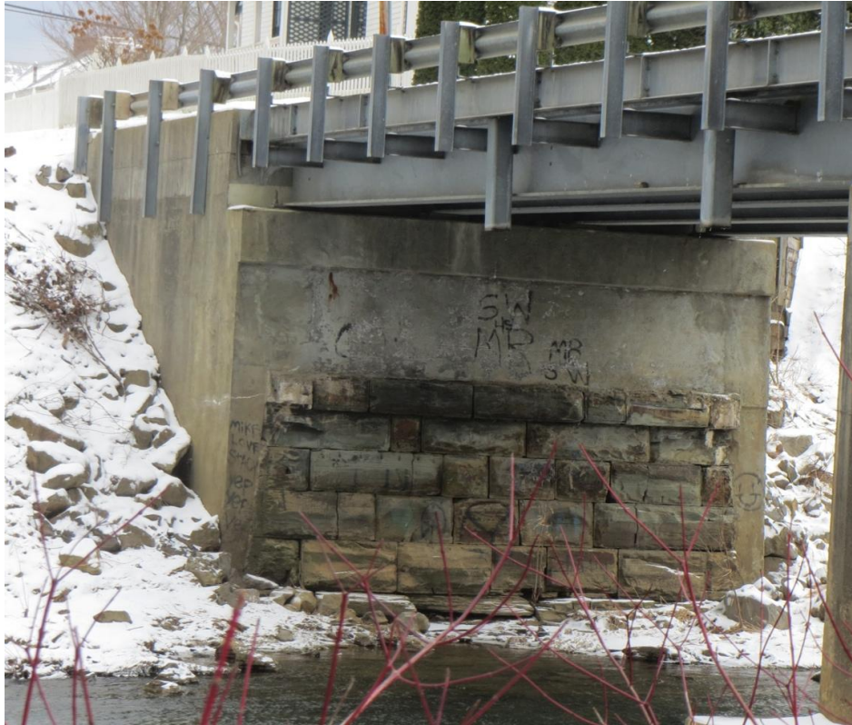
Figure 2.1: Existing Beverly Bridge Abutment (photograph by author, 2014). The concrete abutment for the current bridge was cast around the original masonry structures.
