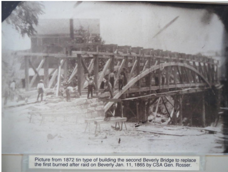
Figure A 6: Construction of the Beverly Bridge, photo courtesy of Randy Allan
