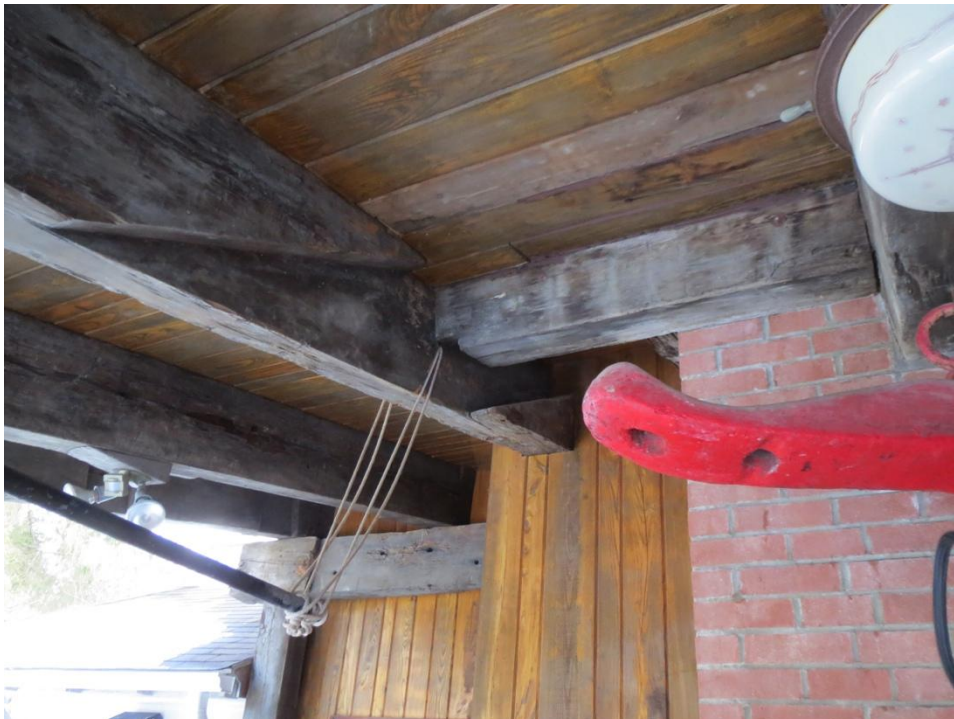
Figure A 13: Salvaged Beverly Bridge Timbers. Note the large transverse cut area, likely the location of an arch and bottom chord intersection
