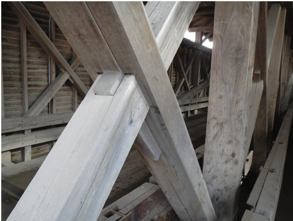
Figure A 30: Diagonal Intersection Detail. A similar connection would be used between the two diagonal elements of the panel resting on the abutments at Beverly.
