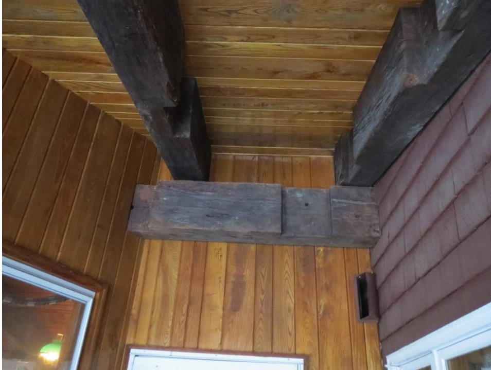
Figure A 12: Salvaged Beverly Bridge Timbers. Note the cut area and single bolt hole of the supporting member.
