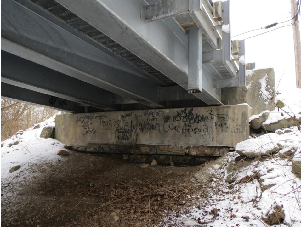
Figure A 4: West Abutment of the Beverly Bridge, mostly obscured by soil and new concrete
