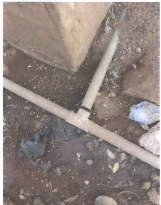
Figure 4-16: Broken distribution pipe (Photo: Deborah Vacs Renwick)
