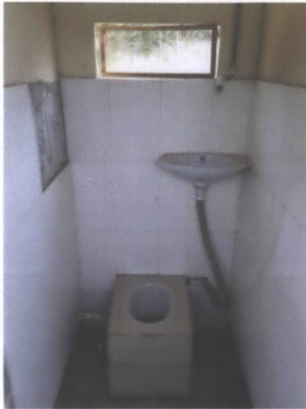
Figure 1-12 Inside of the public Microflush Biofil facility, where the sink connects to the toilet to provide grey water for microflush
