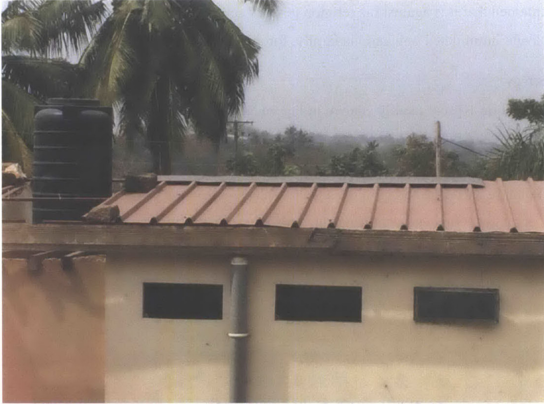
Figure 5-12 The Public MFBB's rainwater collection system and polytank
