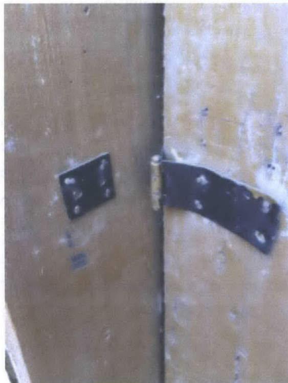
Figure 6-11 Three of six locks have been broken, allowing free use
