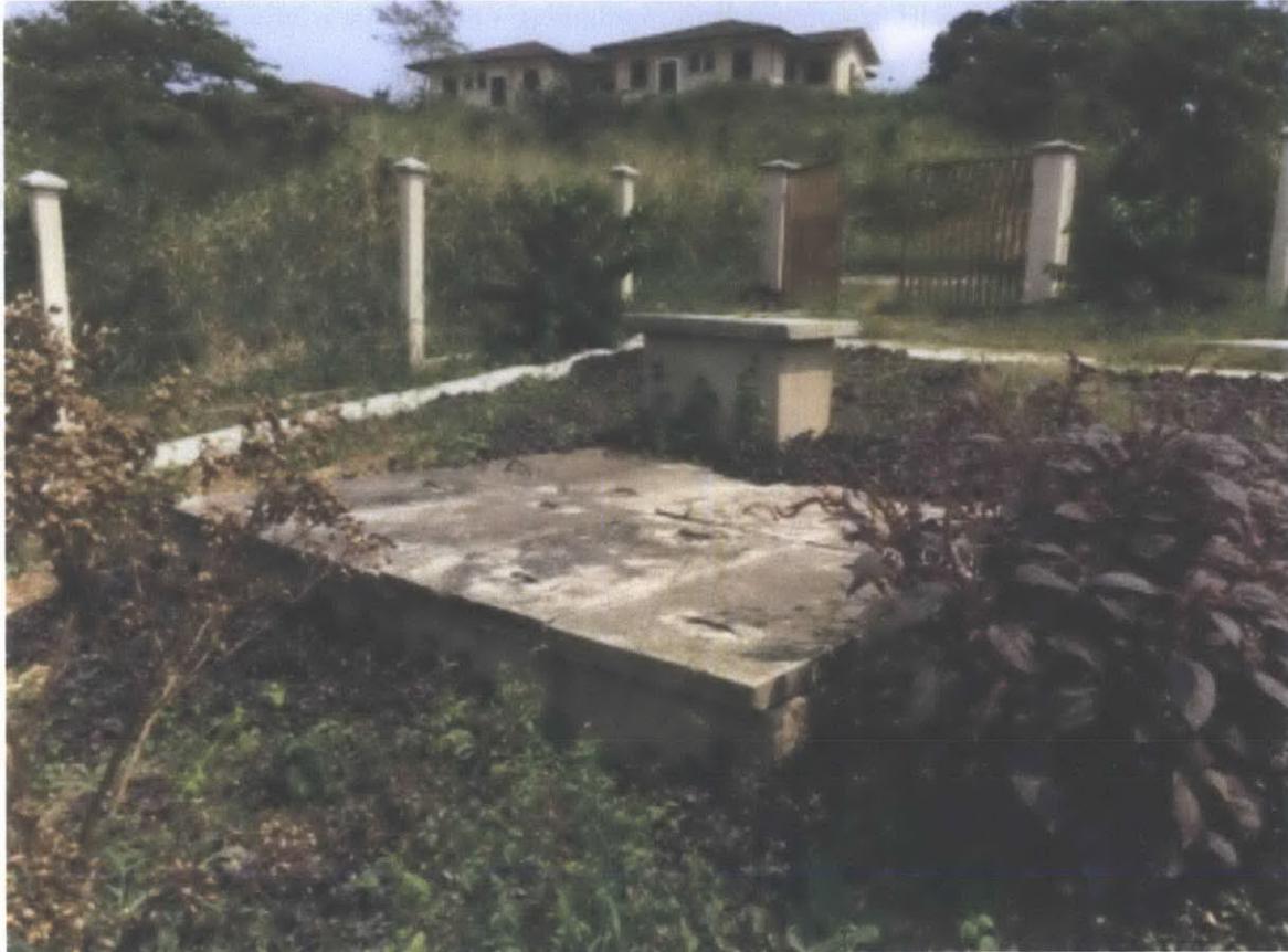
Figure 8-5 Ashesi's primary treatment tank
