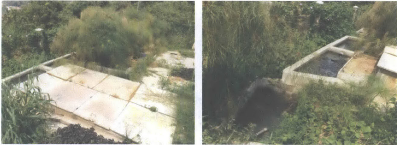
Figure 8-6 Ashesi's tertiary treatment tank uses graphite filters and aquatic vegetation to remove pathogens from the wastewater
