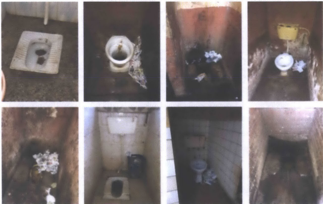
Figure 3-8 A look in on the condition of public sanitation in CTT's service area in Kumasi
