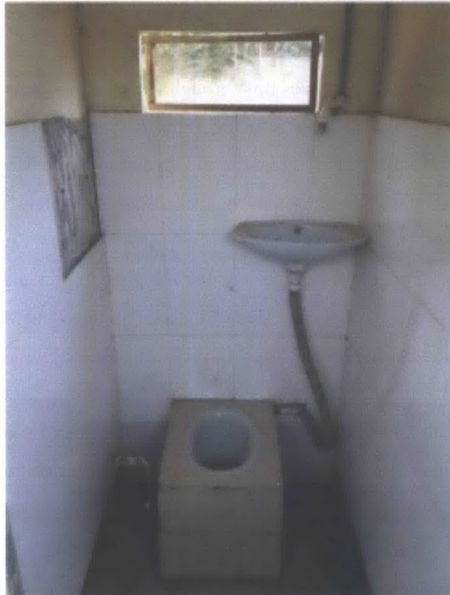
Figure 5-1 Public MFBF facility in Pokuase. Water from the aerator tap used for hand washing is recycled for the next user's flush. Waste is flushed into a tank underneath, where it is composted into a nutrient-rich soil additive through aerobic digestion.
