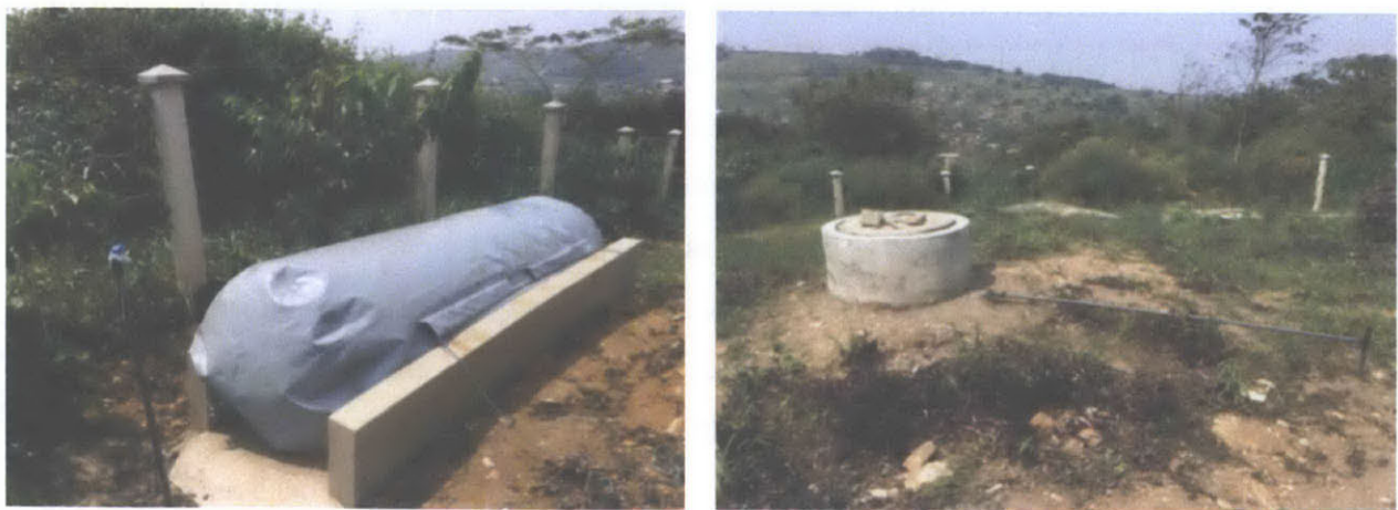
Figure 8-7 The anaerobic digester (right) converts organic material into methane, which is stored in the storage balloon (left) before use as a cooking gas
