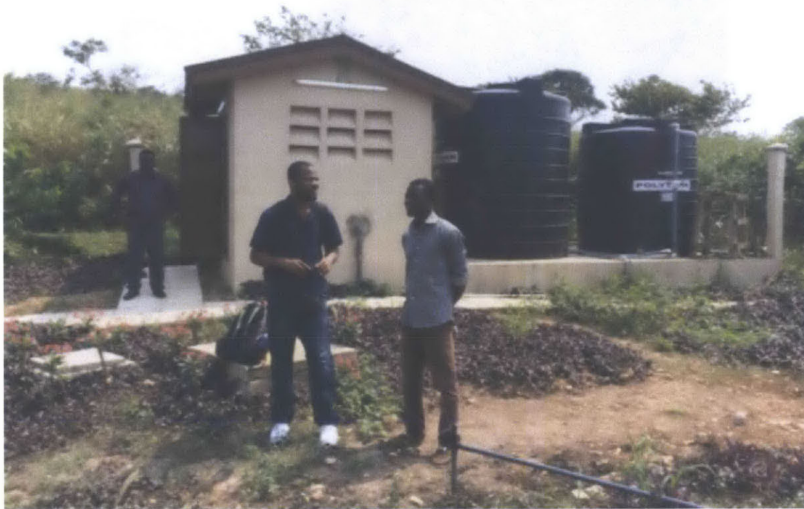
Figure 8-8 The pump house (left) pumps water from tertiary treatment into the chlorination tanks (right) and then sends it to the campus for irrigation.
