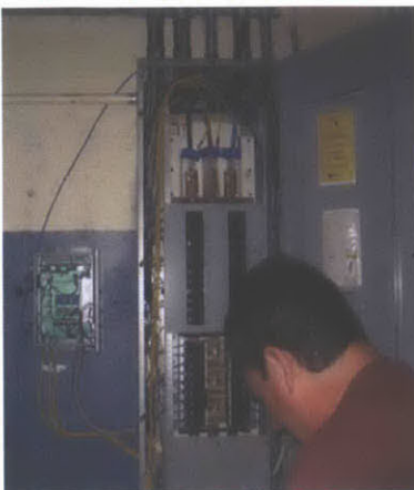
Figure 3-2: Installation of NILM at Cottage Boiler Room panel
