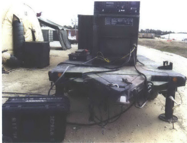
Figure 4-12: DepNILM installation on a CSH generator at Ft. Polk
