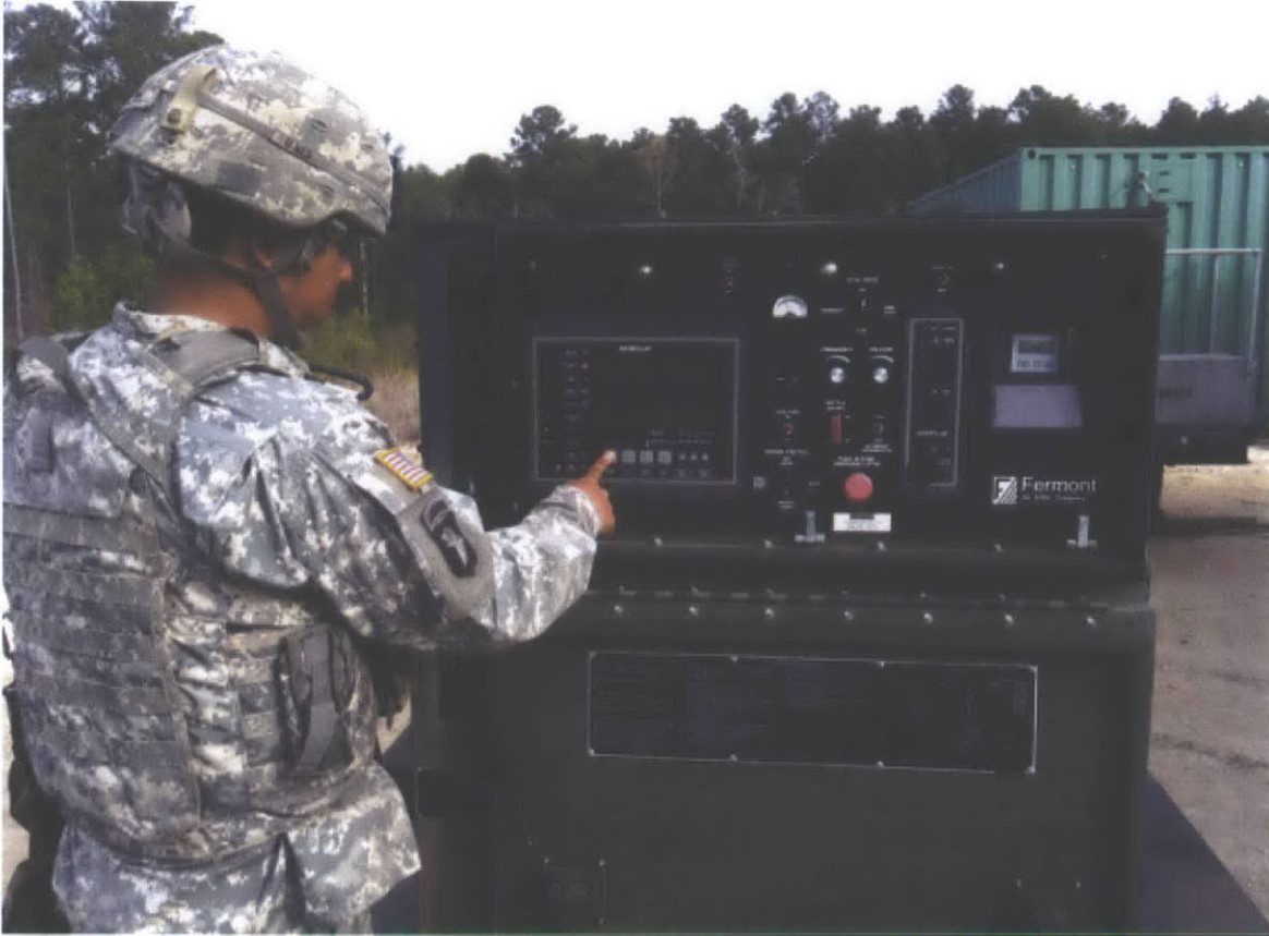
Figure 5-10: Generator Set Control Panel of MEP 807
