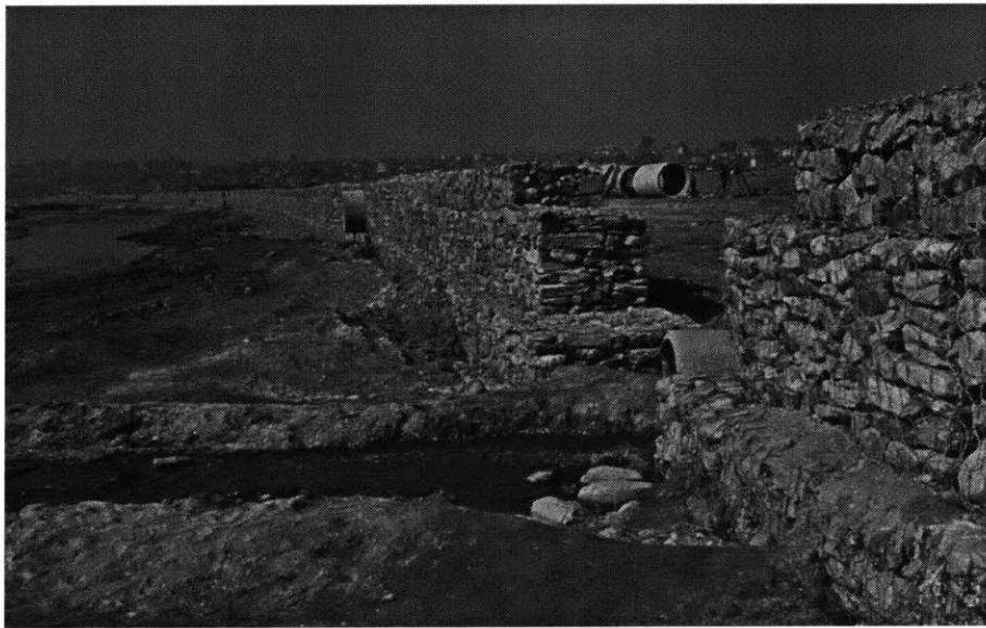
Figure 24: Picture of a large outfall discharging raw sewage into the Bagmati River.
