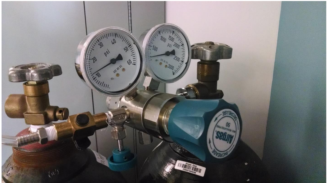
Figure 3-6 A picture of the compressed nitrogen tank and Airgas pressure regulator used to drive the flow
