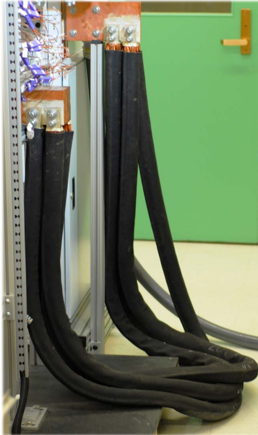
Figure 17: Welding Cables Used to Connect the Negative Electrode of the Power Supply to the Test Section.
