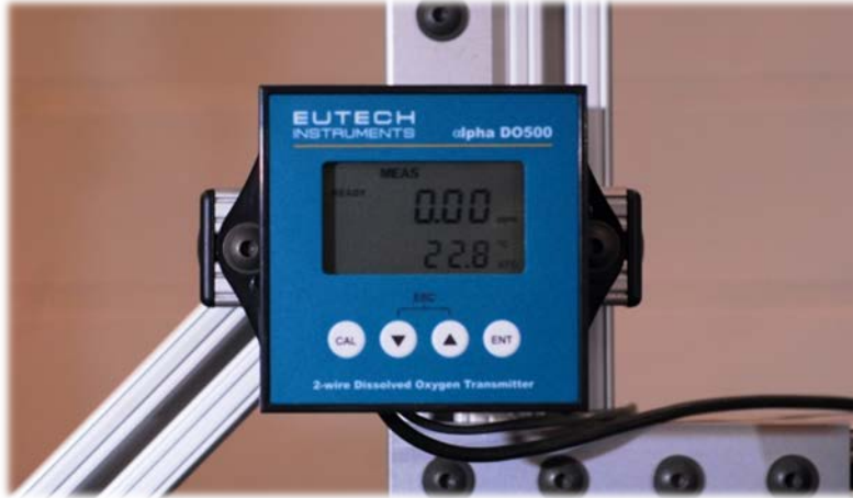
Figure 58: Photograph of the DO Meter Installed in the Facility.
