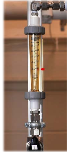
Figure 52: Rotameter Installed in the DO Loop.
