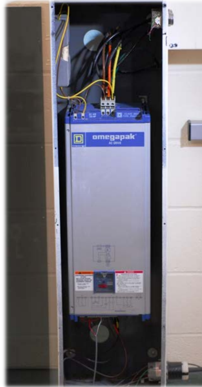
Figure 40: Square D Variable Speed Controller in Metal Enclosure (cover removed).
