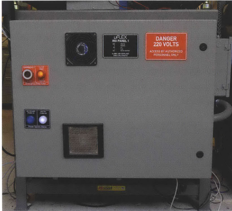
Figure 2.42: The electrical cabinet, closed
