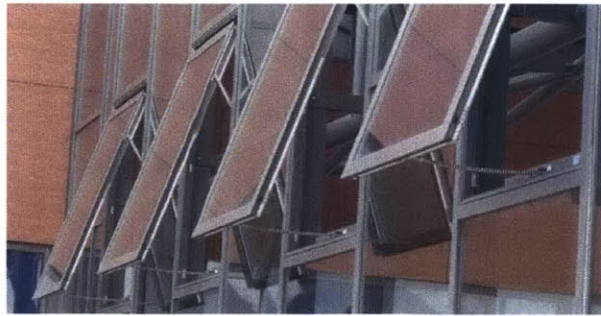
Figure 1-3: Automated windows with hydraulic actuation [7]
