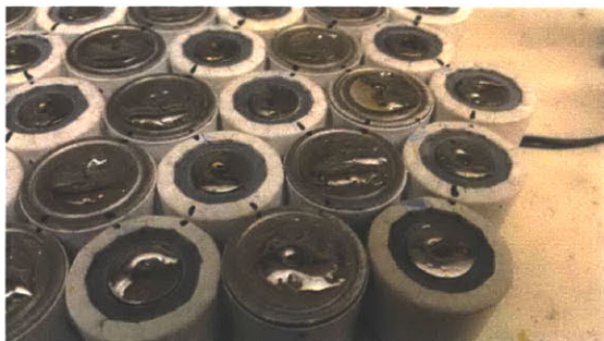
Figure 3-5: Tinned positive and negative terminals of each battery cell
