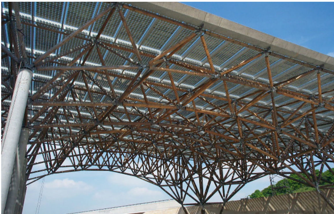
Fig. 3.1.5: Space-truss in regularized round timbers at Doncaster Earth Center.
