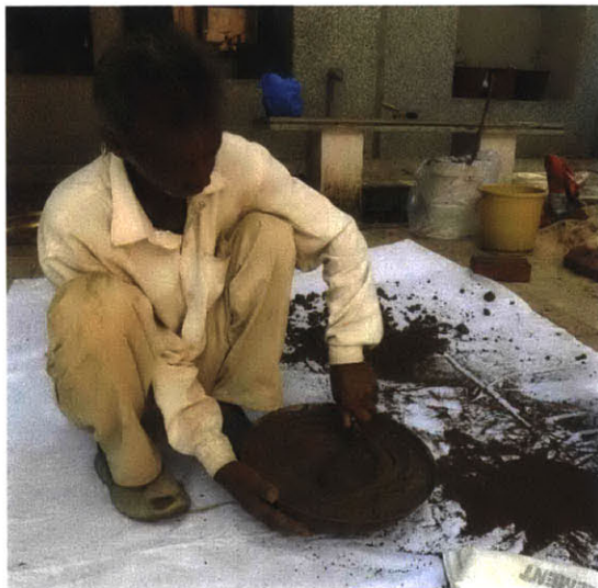
Fig. C.4. Mason mixing mud mortar. Cement mortars were mixed in the same manner.
