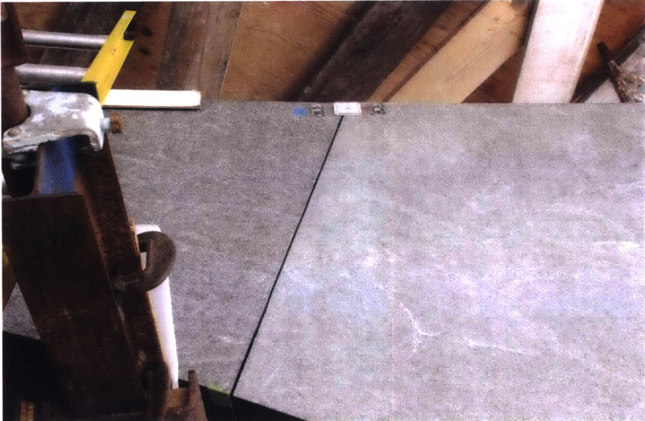
Figure 2.8: Photo of a Crack Monitor in Action (Corentin Fivet)
