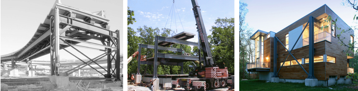
Figure 4: Lexington Big Dig House. Left: the high-way bridge being disassembled, middle: constructing the house, right: the complete building, courtesy of Single Speed Design.
