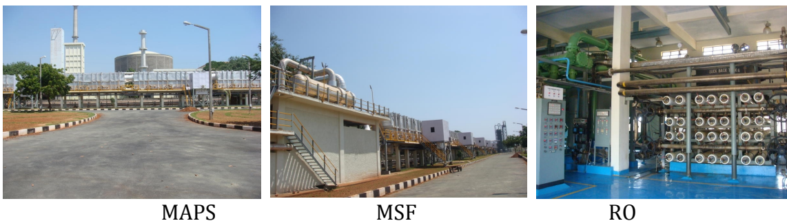
Figure 5.5: Nuclear Desalination Demonstration Plant (NDDP) at Kalpakkam (India) 165
