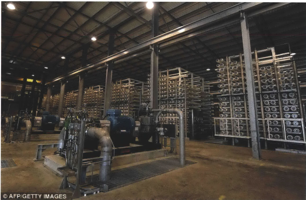
Figure 1-2: Reverse Osmosis Plant [11]
