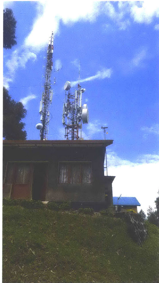
Figure 2.1: Laboratory building for the station. The tall tower is in the background and the smaller tower in the foreground
