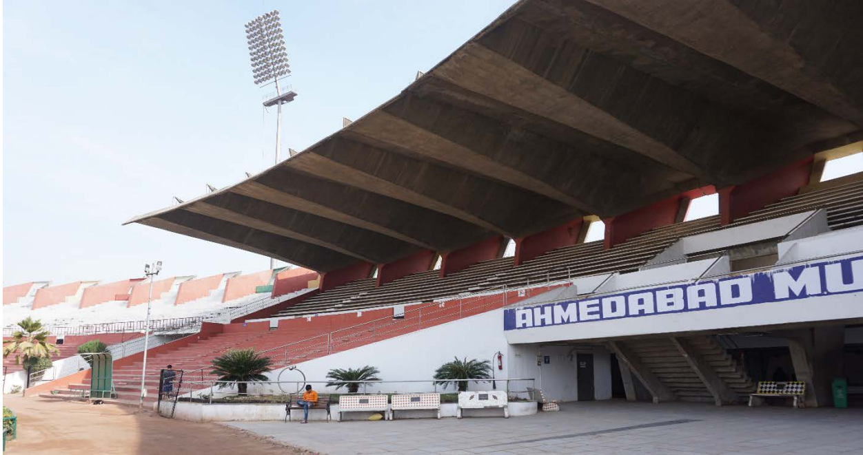
Figure 8 20m span folded-plate roof; Municipal Stadium, Charles Correa and Mahendra Raj, Ahmedabad, 1966
