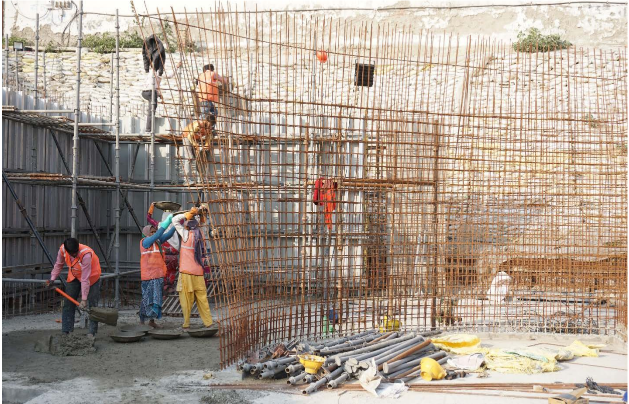
Figure 106 Manual concrete pouring at tower construction site, courtesy of Harsh Vardhan Jain Architects
