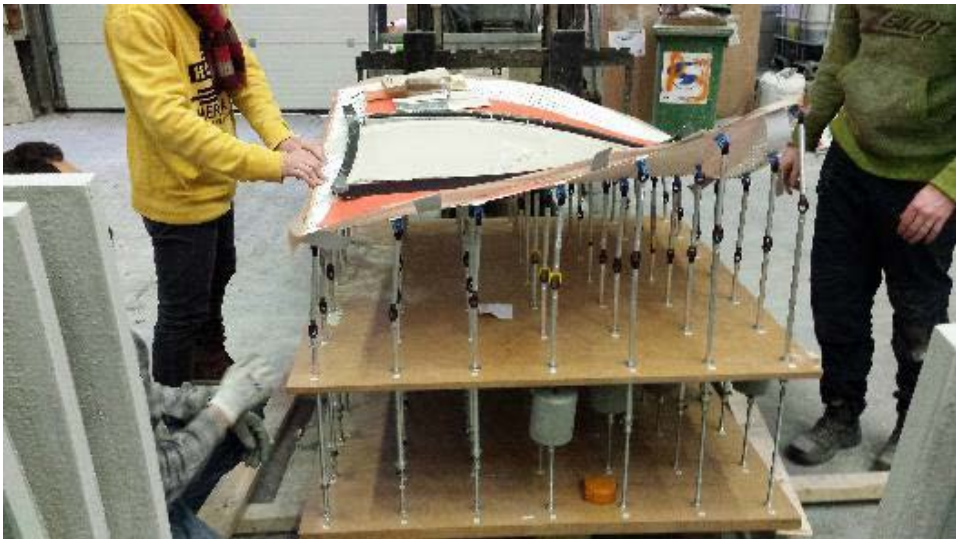
Figure 18 Doubly-curved concrete panel fabricated using adaptive mold system, Delft University of Technology
