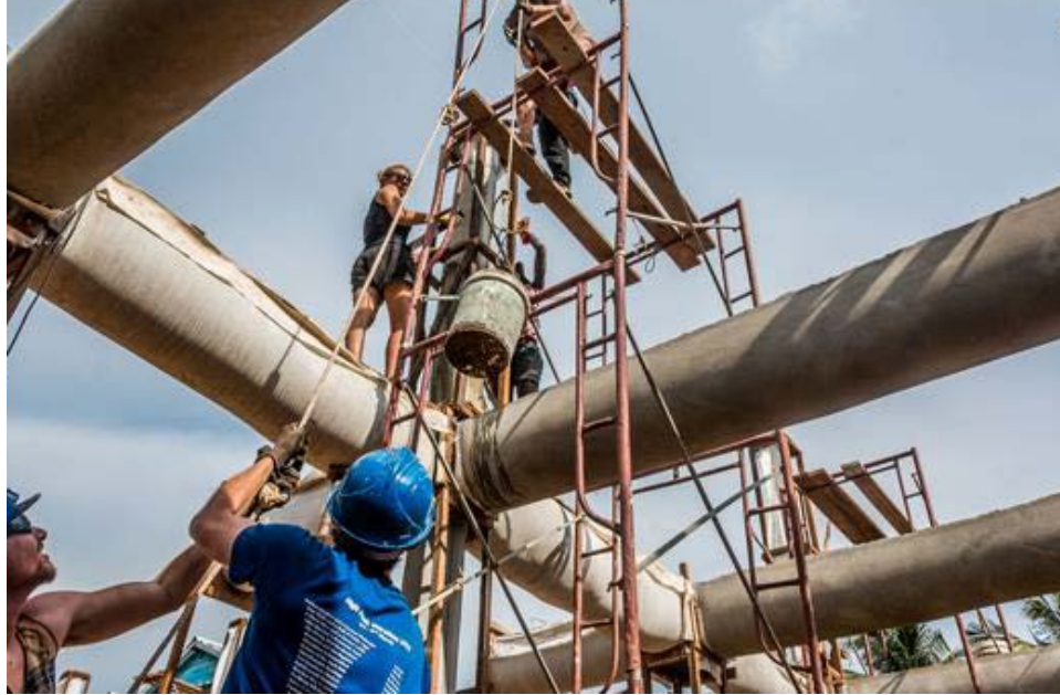
Figure 21 Fabric formwork beams in use at a school in Bomnong L'Or, Cambodia
