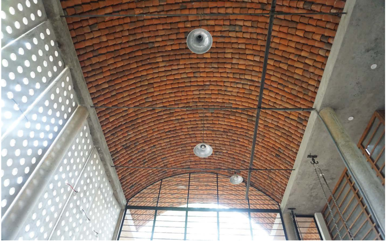
Figure 118 One-way vault built from interlocking conical blocks, courtesy of Anupama Kundoo Architect
