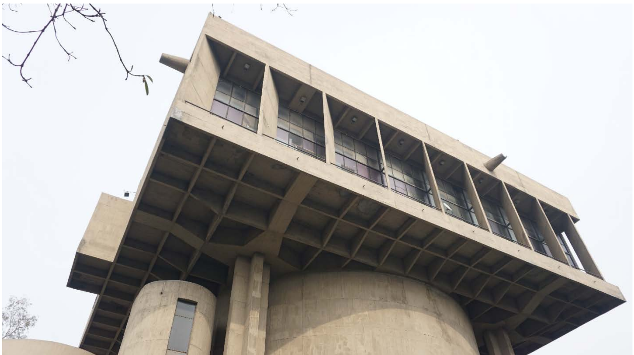
Figure 123 Shaped two-way slab at Sri Ram Centre by Shivnath Prasad and Mahendra Raj, New Delhi, 1969
