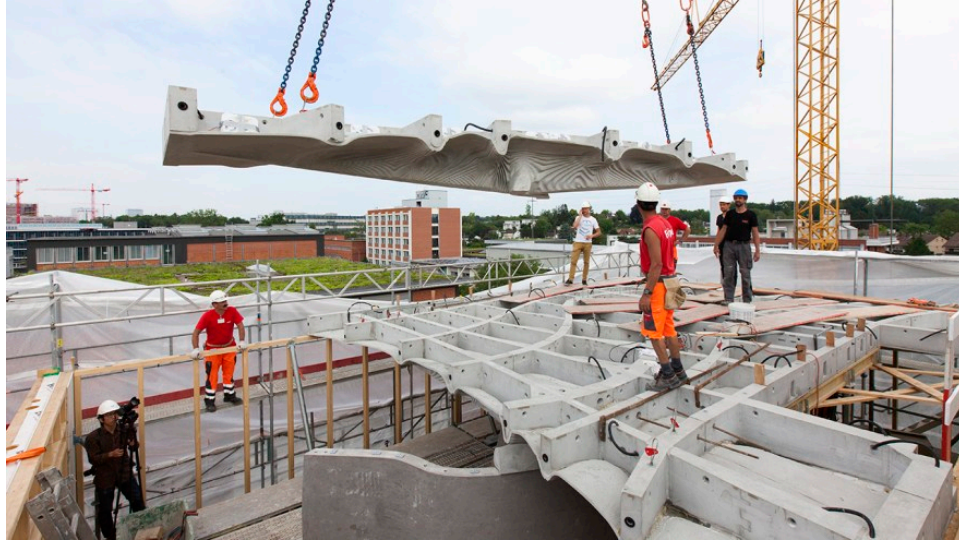
Figure 24 Topology optimized concrete slab built using particle-bed 3D printed formwork, ETH Zurich
