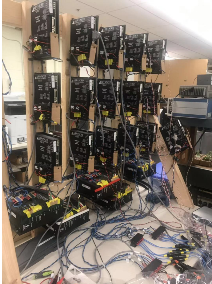
Figure 5-45: Photograph of the rack for power electronics, including DC power supply, power amplifiers, and fuses.
