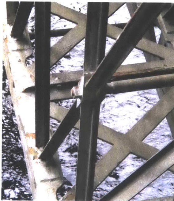
Figure 3.8: Closeup view of Craigellachie Bridge lattice, showing new steel sections and connections
