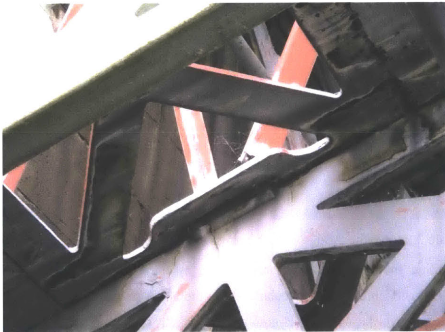
Figure 3.20: Mythe Bridge – corrosion of covering plates (Lane 2017)
