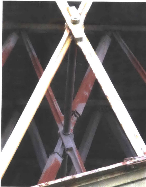
Figure 3.18: Mythe Bridge – bracing mid-span connection, showing original exterior brace and strengthened interior brace, connected by wrought-iron tie encased in cast-iron tube (Lane 2017)
