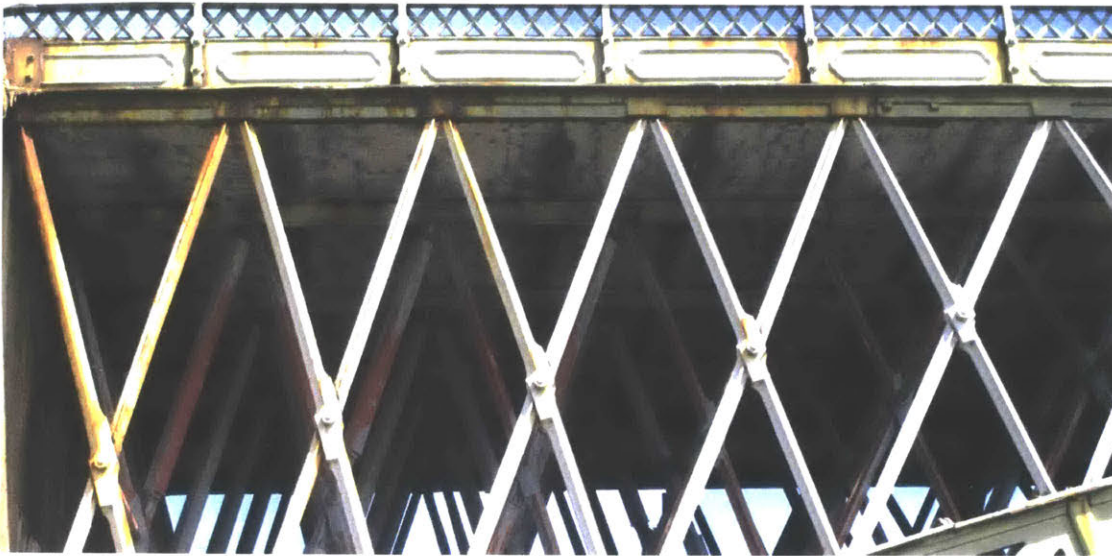
Figure 3.21: Mythe Bridge – deck corrosion along connections between deck plates (Lane 2017)
