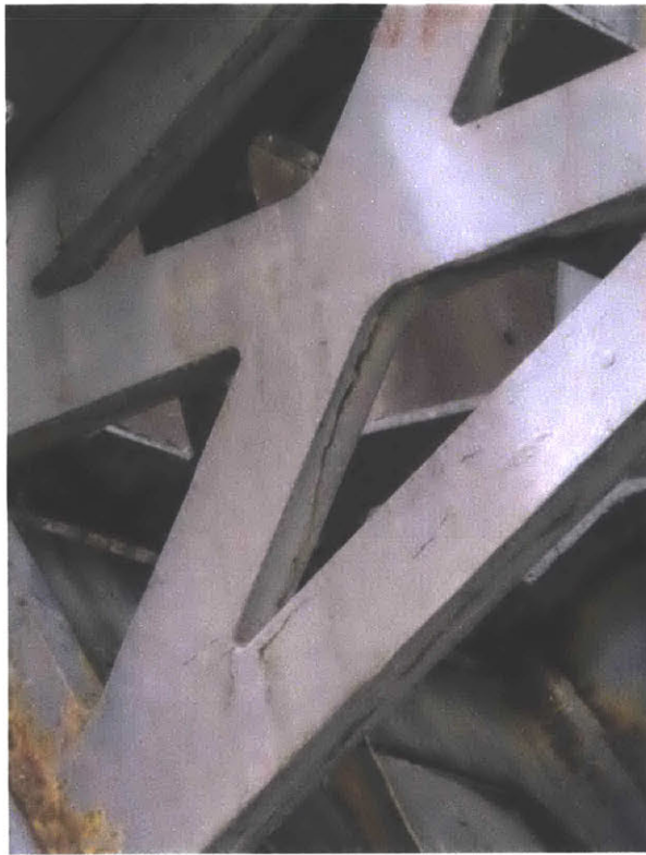
Figure 3.19: Mythe Bridge – longitudinal cracking of rib (Lane 2017)
