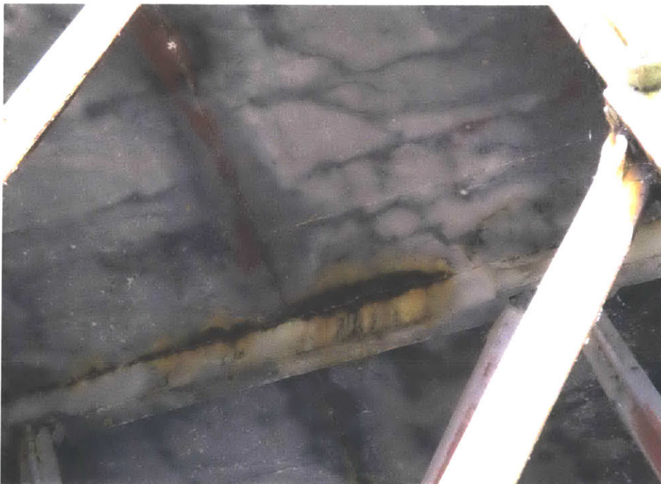
Figure 3.22: Mythe Bridge – deck corrosion along roadway bearer (Lane 2017)
