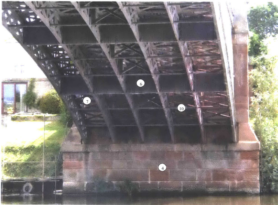
Figure 3.15: Mythe Bridge – viewed from below, showing ribs, connecting plates, covering plates, springing plates, and abutments (Lane 2017)
