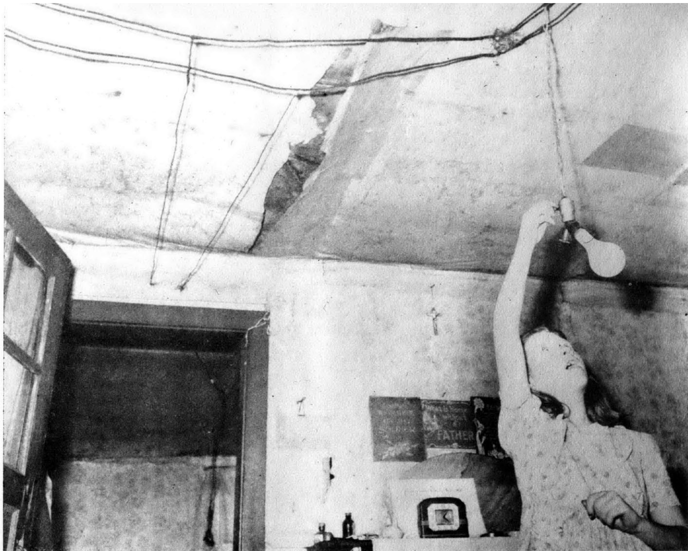
Electrical wiring in much of the company-owned housing is crudely installed and constitutes real fire hazards
