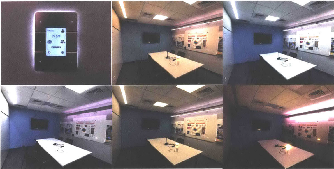
By pressing the button on the wall according to the activity, lights in the meeting room can support people to work effectively and emotionally delighted. Scenes provided: whiteboard focus, F2F collaboration, blue boost, warm boost, A/V, and off/on/auto.
