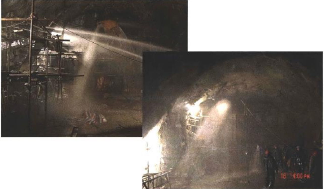
Figure 12 Water burst resulting in flooding, China (private correspondence)
