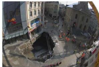
Collapsed area at the surface
