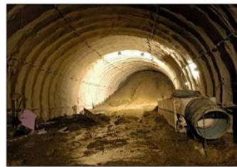
Aspect of the front after collapse (ingress of soil and water)
