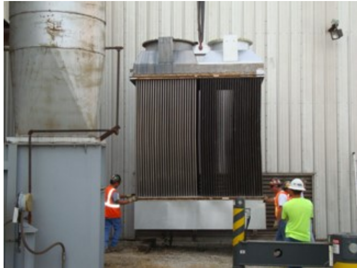
Figure B-4: The recuperator used in Molycop's USA plant
