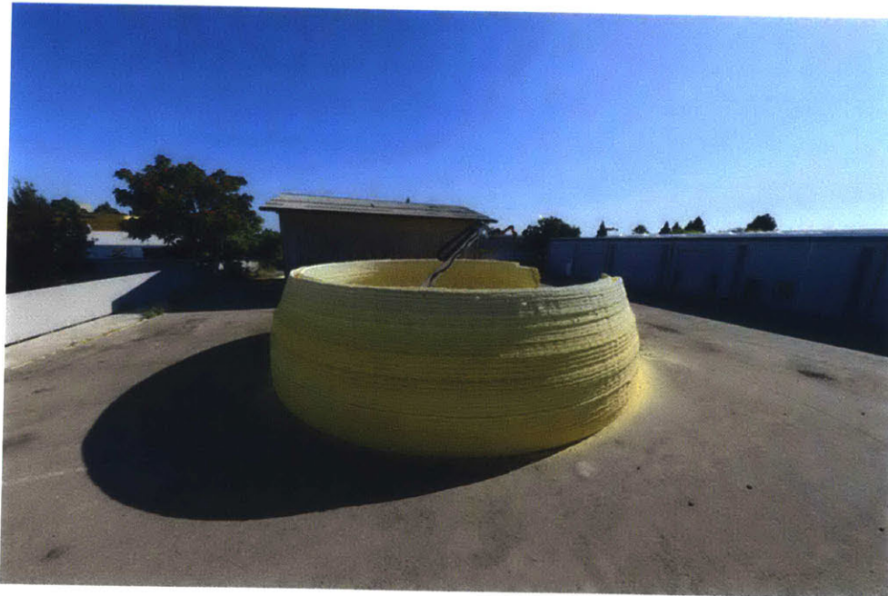
Figure 20: Overall test conducted in July 2016, 13.5 hour total print time, 14.6 m diameter, 3.7 m tall, with 306 layers. Walls had double curvature and used no support material.
