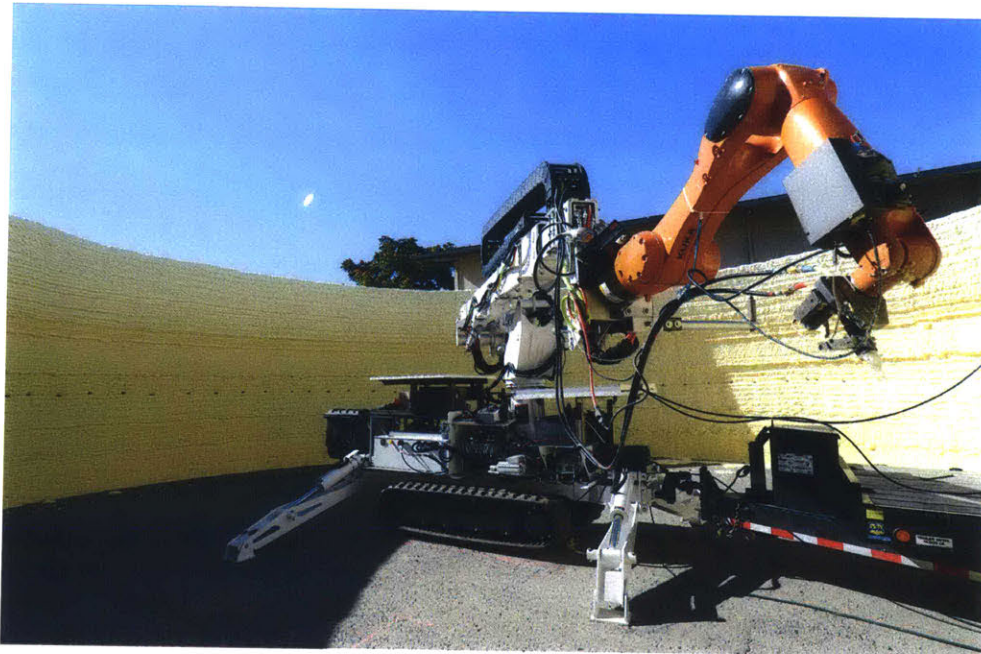
Figure 2: The Digital Construction Platform v.2 with spray foam end-effector and trailer attachment, during a large-scale print. The orange arm is a KUKA KR10 R1100, the white vehicle is an Altec AT40GW aerial boom truck.
