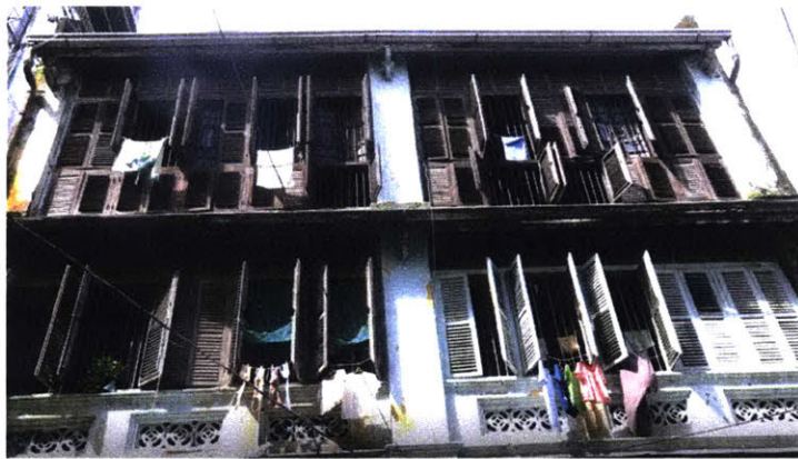
Building on 21 st Street, Yangon in the Chinatown with 1900 style Chinese shutters (Bob Percival)
